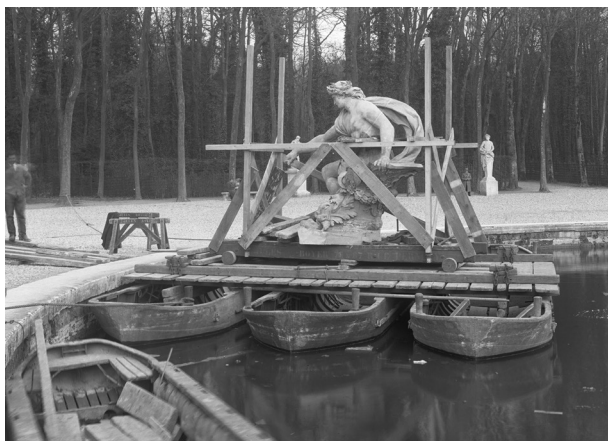
Disassembly of the set of sculptures for it to be restored in 1923-1927 © Archives of the Palace of Versailles
