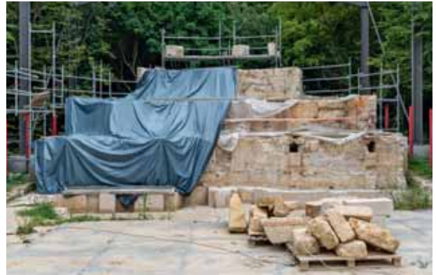
Work in progress to restore the Water Sideboard Fountain © Palace of Versailles, S. Giles
