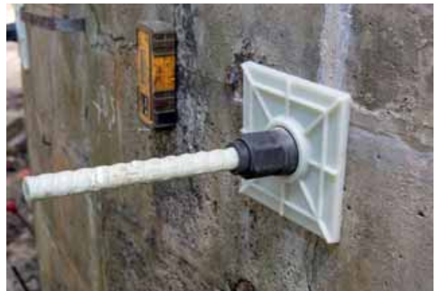
Tie rod on the back of the Water Sideboard Fountain's stonework and sensor to monitor stability in the fountain and its foundations © Palace of Versailles, D. Saulnier
