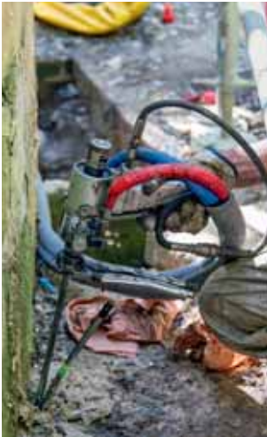
Resin injections beneath the Water Sideboard Fountain's stonework © Palace of Versailles, D. Saulnier
