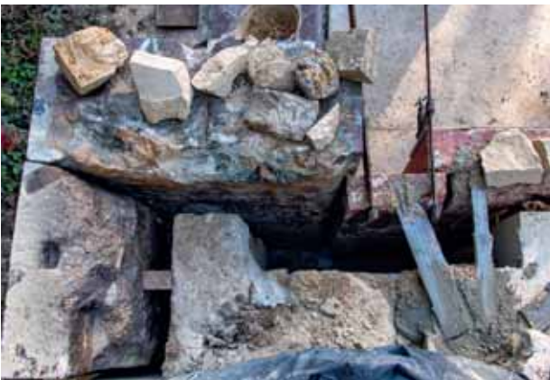
Filling blockouts between the stonework structure and cladding marble after fixing the fasteners © Palace of Versailles, D. Saulnier
