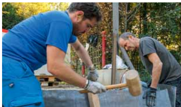
Cutting back the lead for the lining on the lower basin © Palace of Versailles, D. Saulnier
