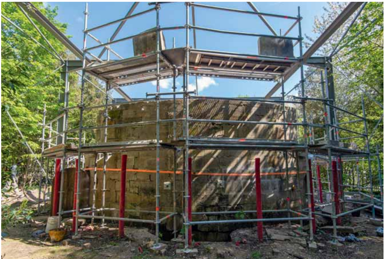
Work in progress to restore the Water Sideboard Fountain, stonework at the back of the fountain © Palace of Versailles, D. Saulnier
