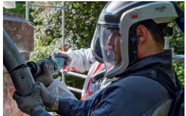
Adjusting the lead piping on the back of the structure © Palace of Versailles, D. Saulnier
