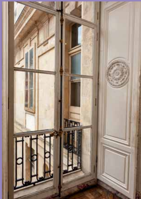
View from the first floor of the private chambers © Palace of Versailles, T. Garnier
